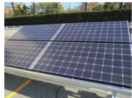
[太陽光発電実習装置]
